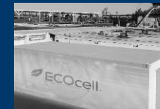
Battery Storage Systems
