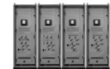
Substation controls Grid protection, monitoring, and automation at the point of interconnection
