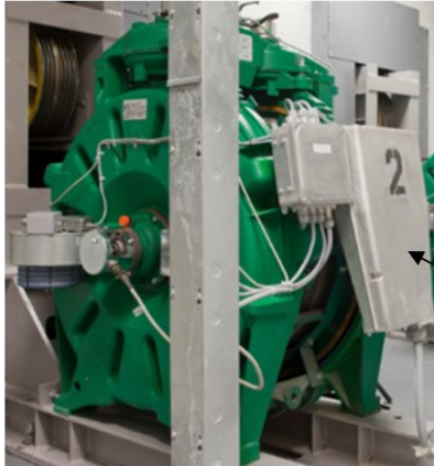
Motor Drives Control Panel
