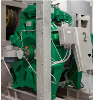
Motor Drives Control Panel
