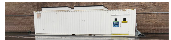
Zinc treatment system.
