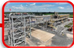
Capture Facility (CO 2 compression and conditioning)
