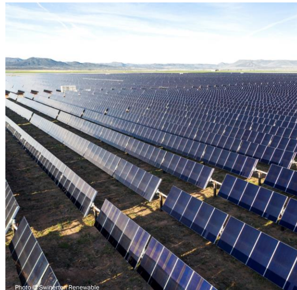
Photo © Swinerton Renewable
