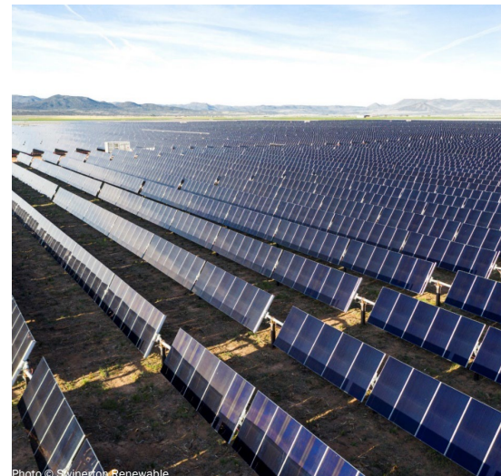
Photo © Swinerton Renewable
