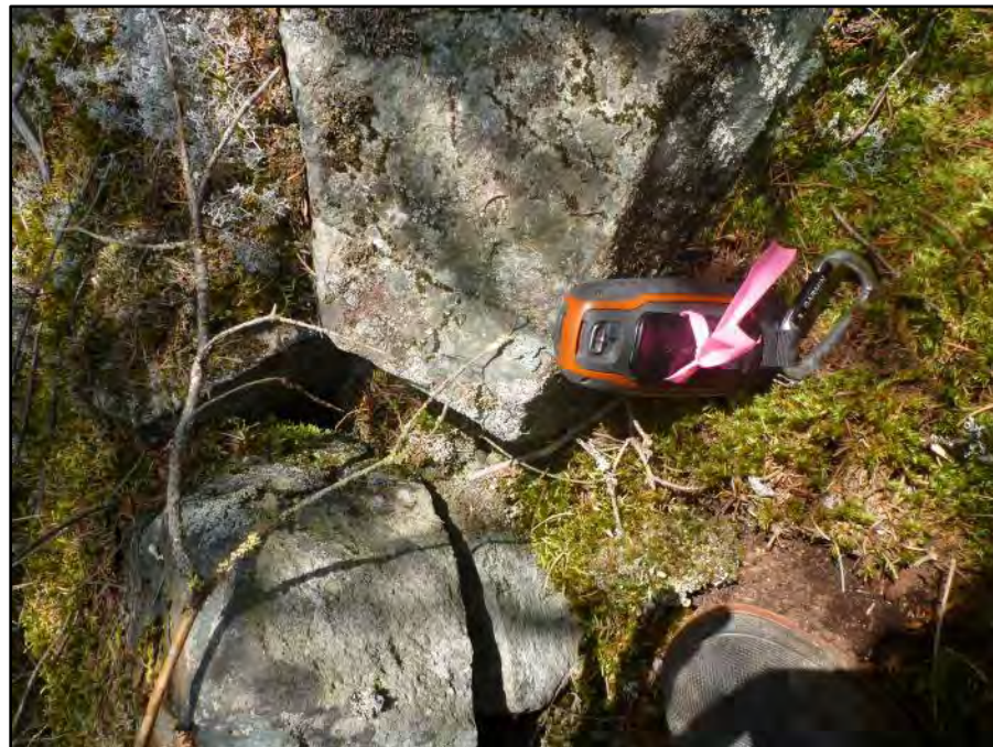
Photo 7: Crevice observed at 98med
