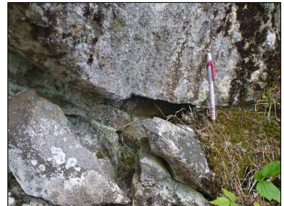
Photo 12: Crevice observed at 115lo
