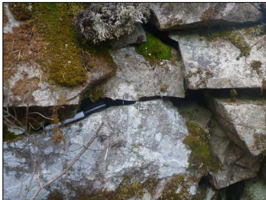
Photo 14: Crevice observed at 117lo
