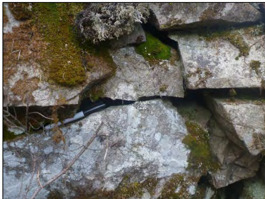
Photo 14: Crevice observed at 117lo
