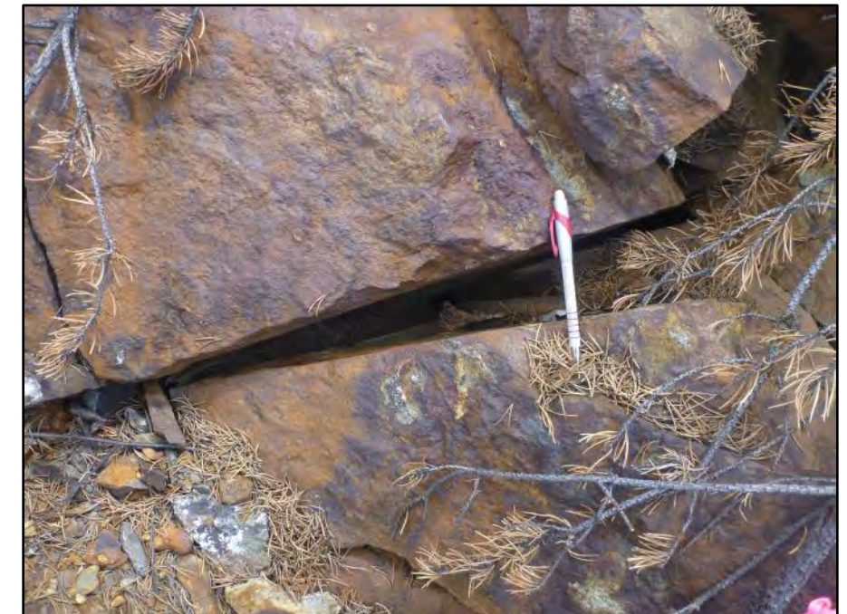
Photo 17: Crevice observed at 100med
