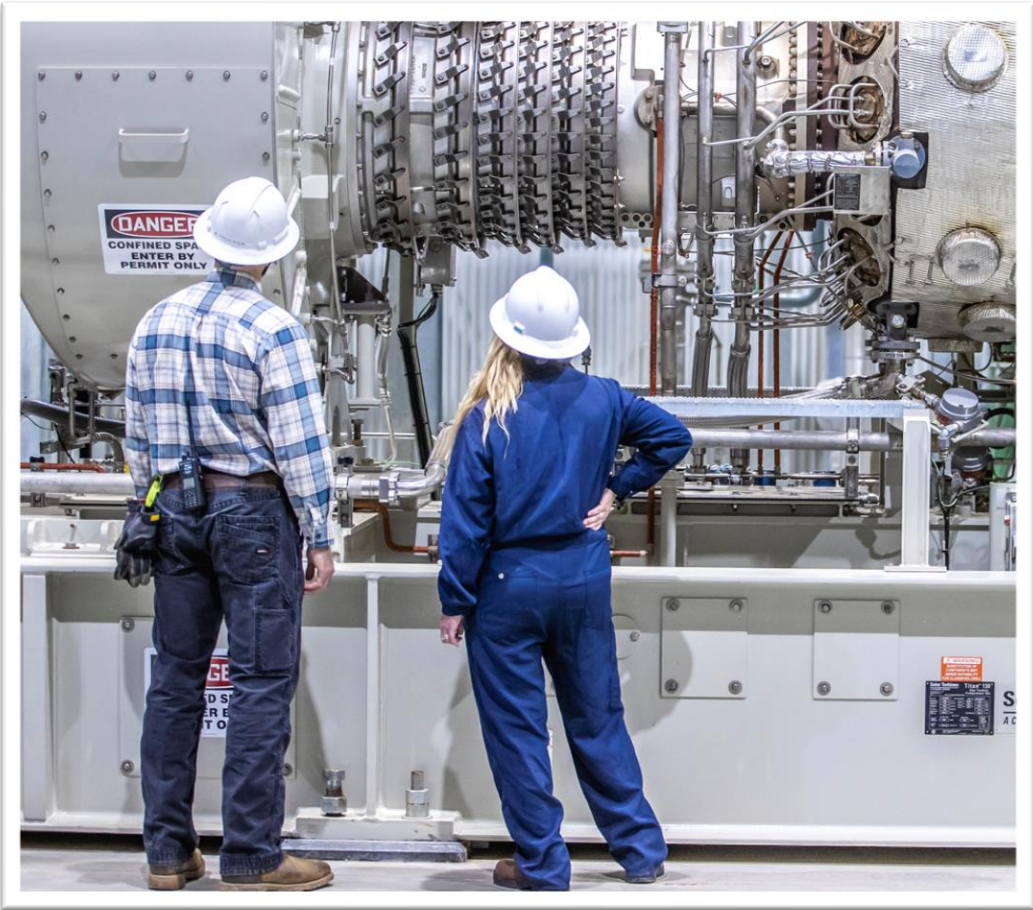
Transco Compressor Station 175 in Virginia
