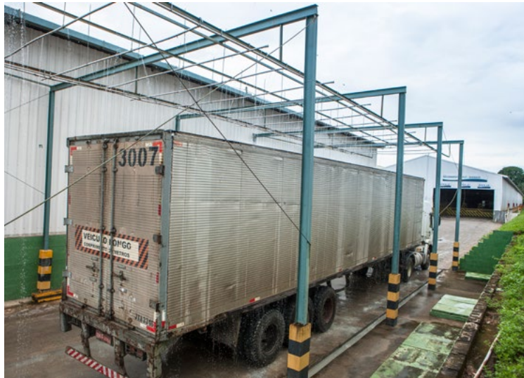
Rainwater reuse system in Manaus, Amazonas, Brazil, that is used to test water tightness on trucks
