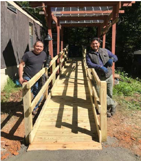
Crane ChemPharma & Energy associates based in Marion, North Carolina, building a wheelchair ramp as part of an effort by Pleasant Gardens Baptist Church to help the disabled in the area.
