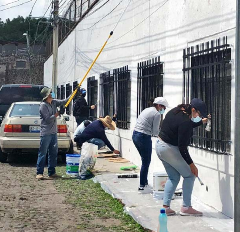
Crane Payment Innovations associates in Queretaro, Mexico, helping with building maintenance at the Centro de Protección de Ancianos.
