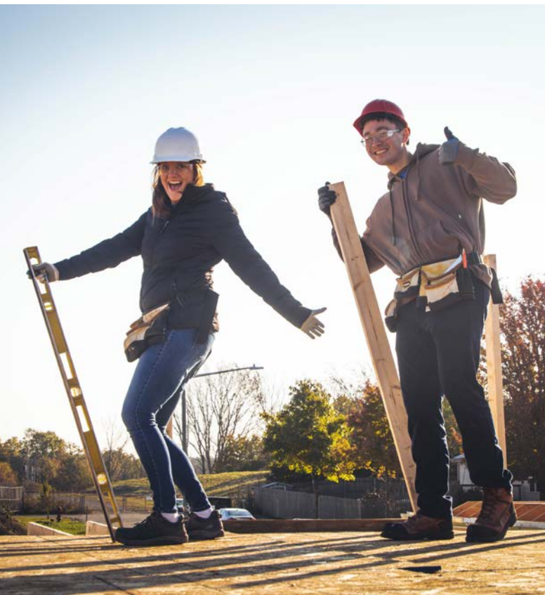
Crane Composites associates in Joliet, Illinois, working with Habitat for Humanity to build affordable housing.
