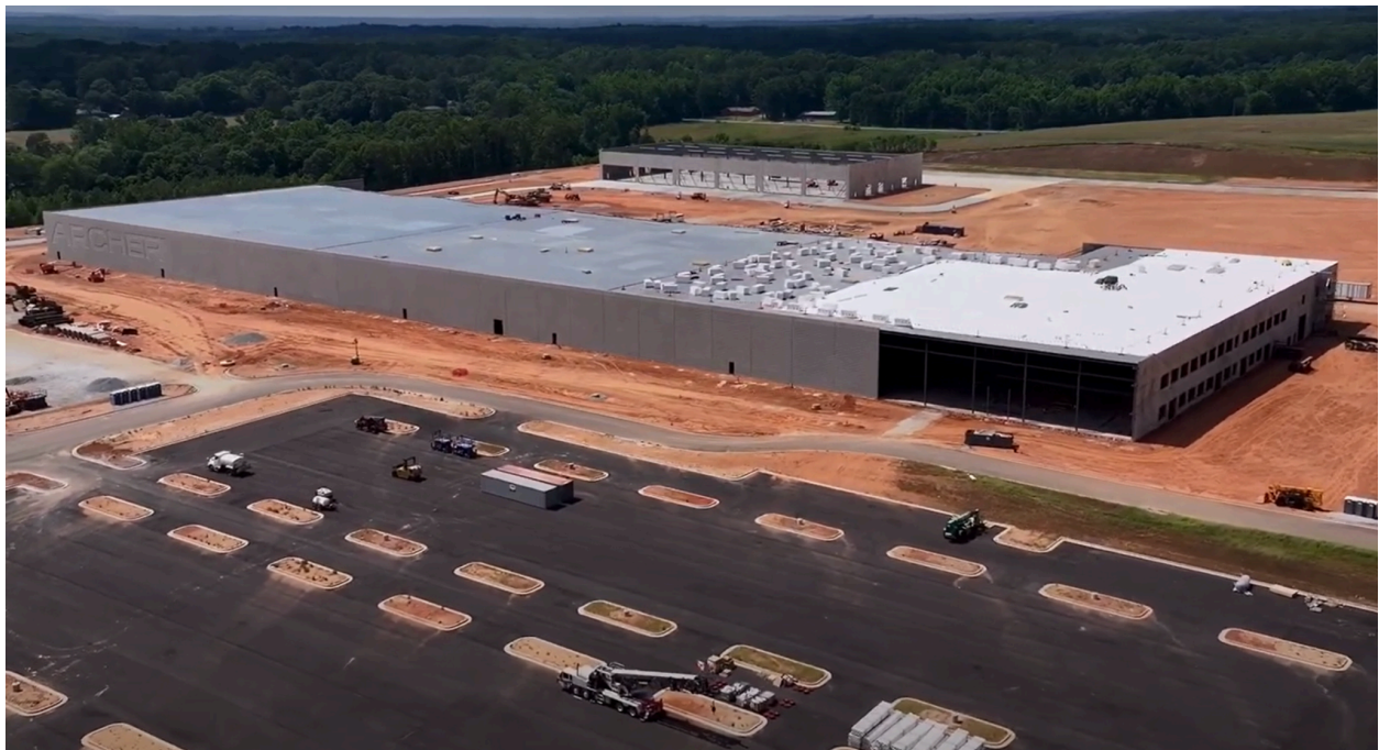
Image above shows latest progress on the construction of Archer's high-volume manufacturing facility in Covington, GA which connects to the Covington Airport
