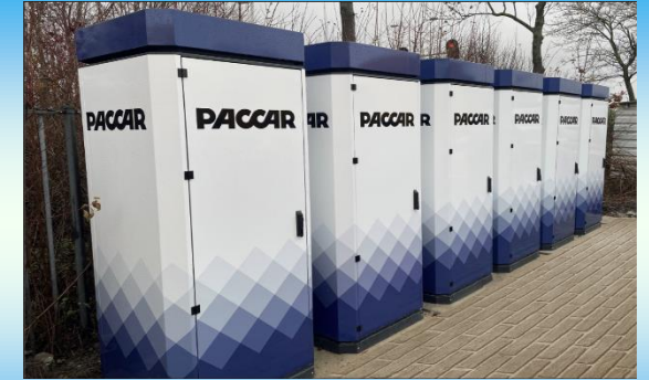
PACCAR Energy Storage System
