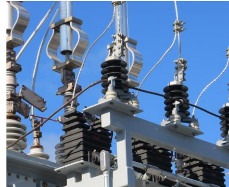
Utility joints, transition joints, terminations and junction boxes
